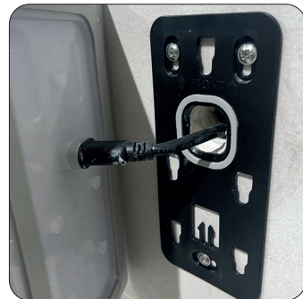
Data cable connection
