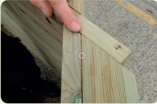
Top view of Shelving Support in place
