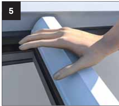
5 Using the heel of your hand, push down on the top cap to engage the clips, working from ridge to eaves. Ensure the rubber gaskets are full compressed for a watertight seal. NOTE: on longer bars it may be necessary to use a soft mallet and timber block
