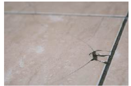
Fill any gaps or recessed grout lines to make the surface completely flat
